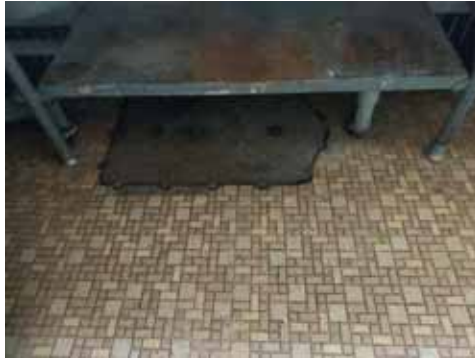
6.8: In-floor grease interceptor
