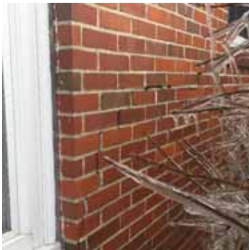
2.6: Step cracking from lower window sill to adjacent higher window sill
