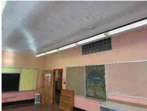
5.11: Typical classroom lighting
