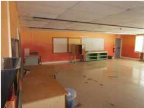
3.32: Delaminated flooring on slab at modulars
