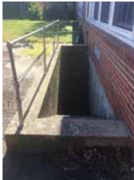
2.26: Noncompliant railings at stair to boiler room
