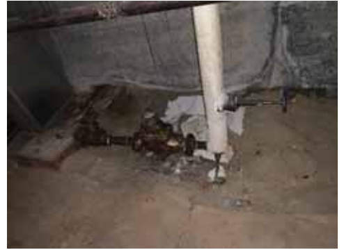
6.9: Domestic water service & meter
