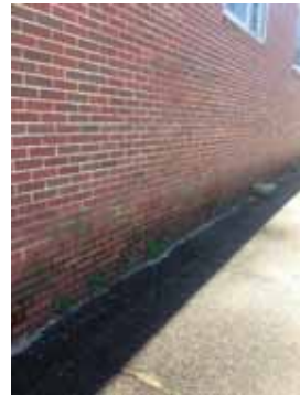
2.33: Algae growth at bottom of wall
