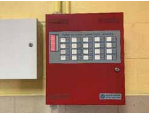
5.19: Fire alarm control panel
