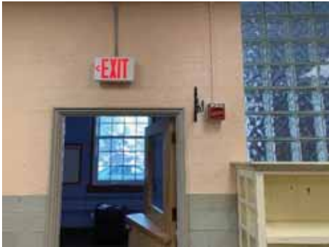
5.17: Lit exit sign
