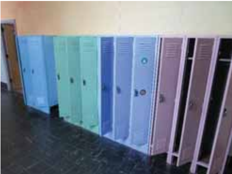
3.26: Metal lockers in poor condition
