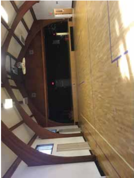
Figure 21: Multi-purpose room. Note no paper under floor.
