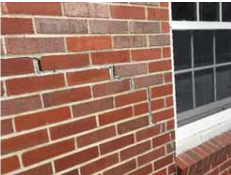
2.5: Typical cracked brick and mortar joint at corner; this condition occurs in numerous locations
