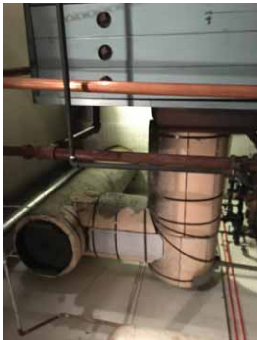
Figure 3: Pink boiler breeching insulation. Note assumed grey boiler breeching insulation at top
