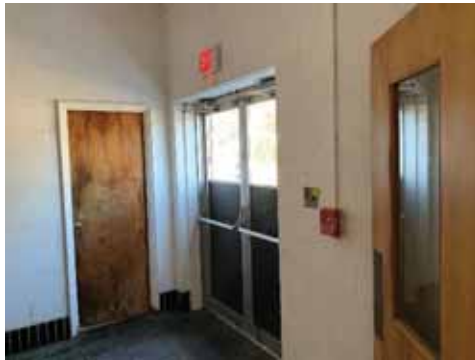
5.20: Fire alarm pull station
