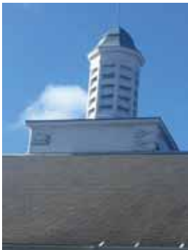
2.8: Cupola requires repainting
