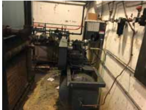
4.17: Pneumatic ATC compressor
