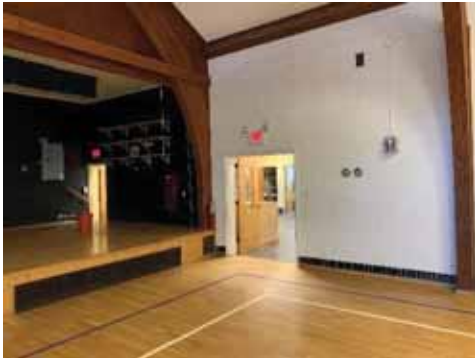
5.18: Exit light with emergency light heads
