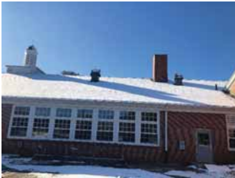
4.13: Roof exhaust ventilators
