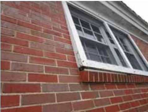
2.34: Damaged, displaced mesh wood-framed screens
