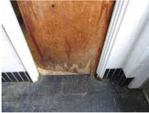
3.2: Deteriorated toilet room door to toilet
