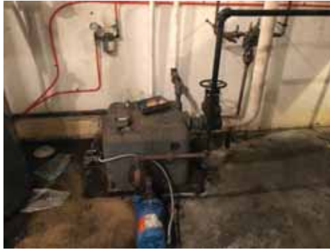
4.2: Existing condensate receiver and pump
