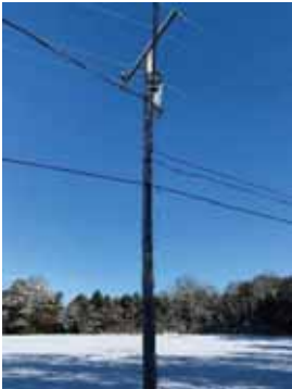
5.2: Modular building riser pole
