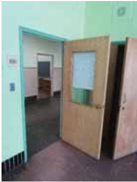
3.13: Noncompliant door hardware
