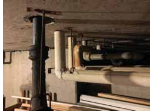
6.12: Water piping in crawl space
