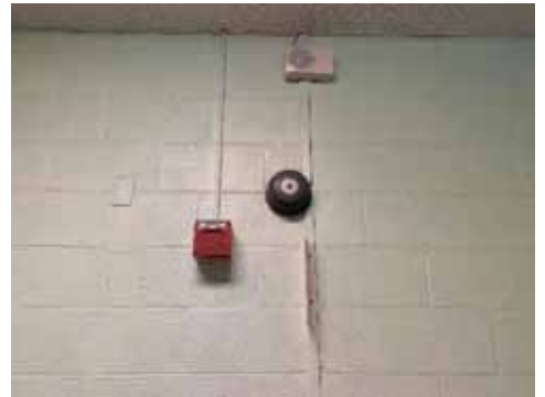
5.21: Fire alarm horn/strobe
