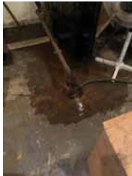
6.17: Boiler Room drain clogged
