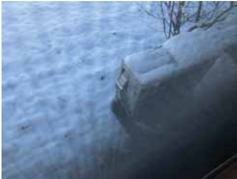
4.16: Modular classroom – outdoor condenser unit
