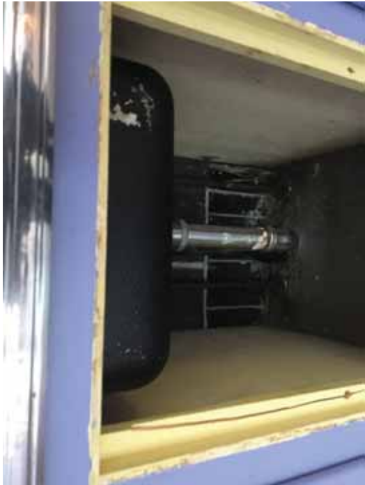
Figure 17: ACM black sink undercoat
