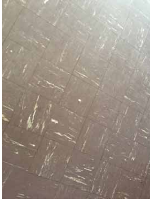
Figure 16: ACM 9" x 9" purple streaked floor tile (Mastic is not asbestos)
