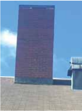
2.9: Brick chimney and cap require repair
