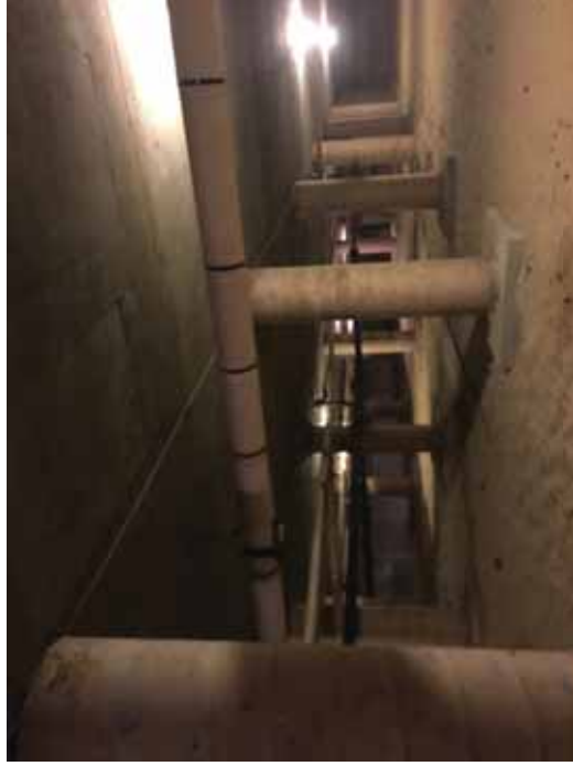
Figure 2: ACM pipe insulation/fittings in basement crawlspace
