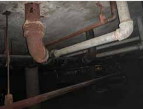
6.16: Galvanized steel vent
