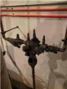
6.10: Make-up water backflow preventer
