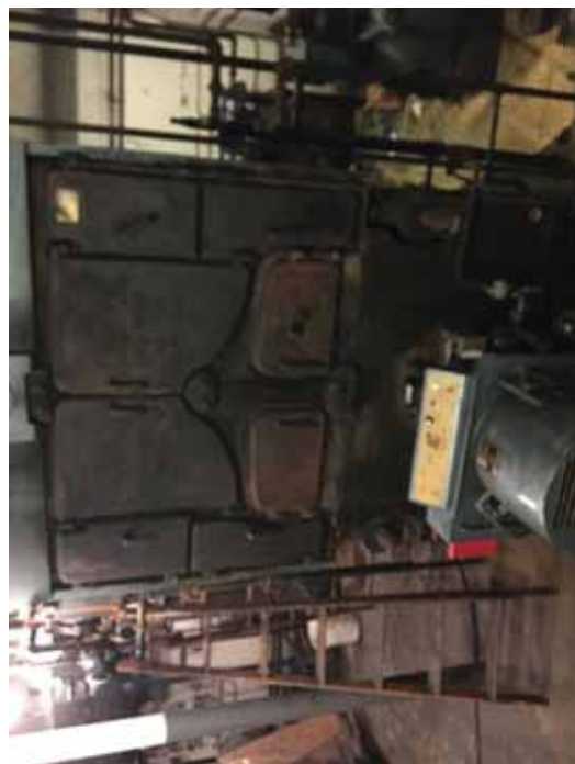
Figure 4: Boiler unit (in operation, assumed ACM components inside)
