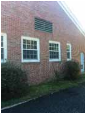
2.40: Damaged, aged kitchen louver
