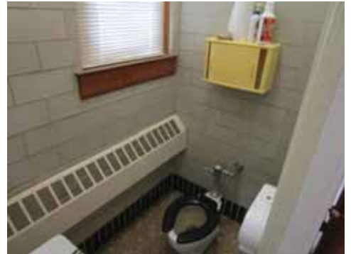
3.10: Noncompliant toilet rooms throughout the building
