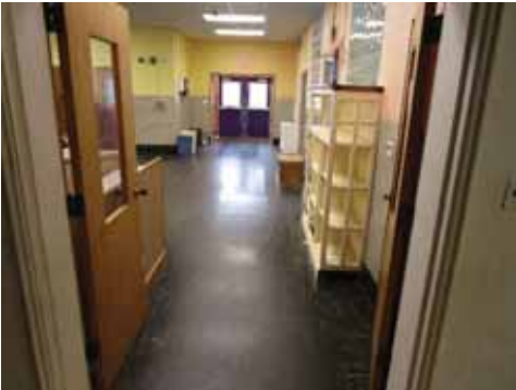
3.7: Asbestos floor tile in lobby area
