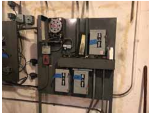
4.20: Pneumatic control panel
