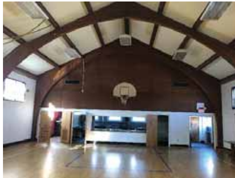
4.11: Cafetorium sidewall supply diffusers
