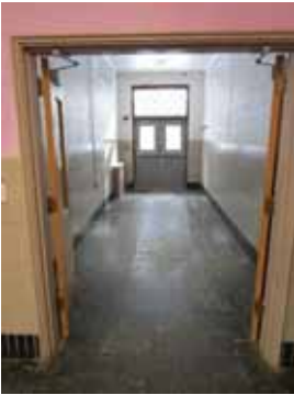
3.35: Double 30" doors do not comply to egress requirements
