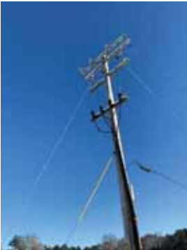
5.1: Main building riser pole
