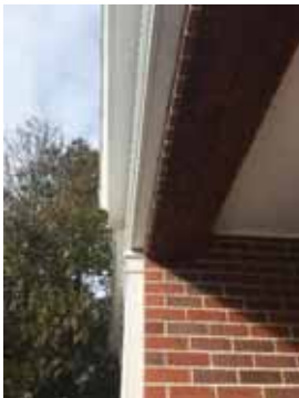
2.4: Typical rusted steel lintel to be scraped, primed and painted
