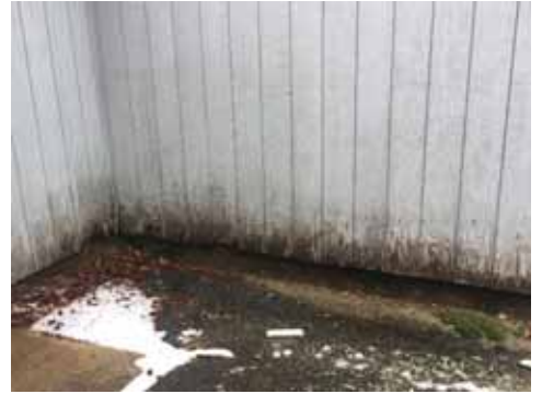
2.20: Deteriorated wood siding at modulars
