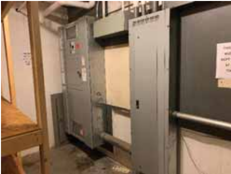
5.5: Main circuit breaker switchboard
