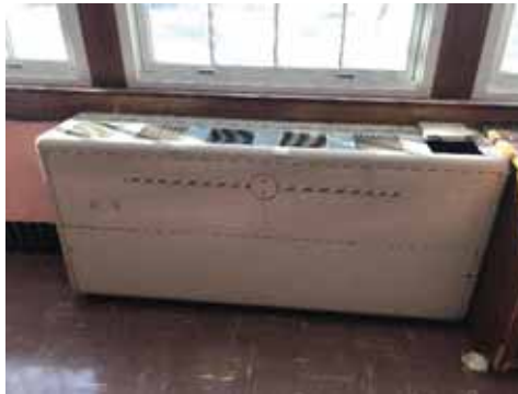
4.8: Classroom unit ventilator
