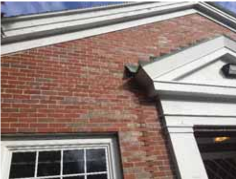
2.1: Stained and deteriorated mortar at front entrance pediment
