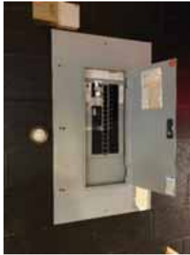
5.8: Typical panel in gym area
