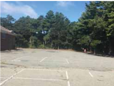
1.4: Bituminous pavement at rear of school in poor condition
