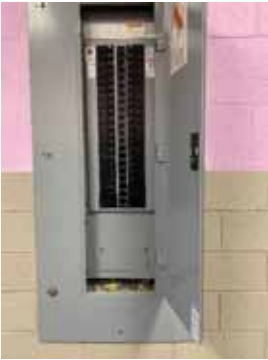
5.7: Typical panel in corridor
