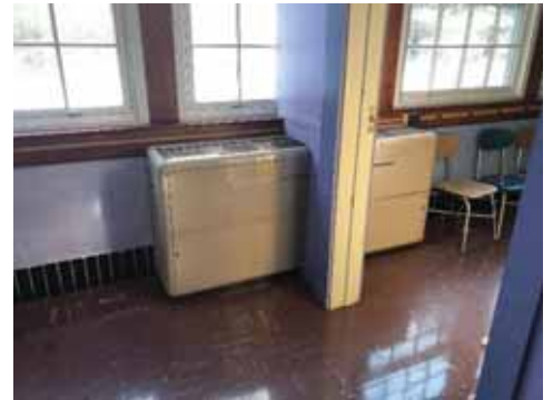
4.9: Classroom unit ventilator installed between two classrooms
