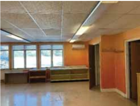
5.13: Modular classroom lighting
