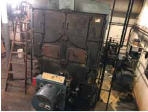
4.1: Existing steam boiler
