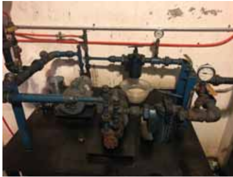
4.5: Boiler fuel oil pumps
