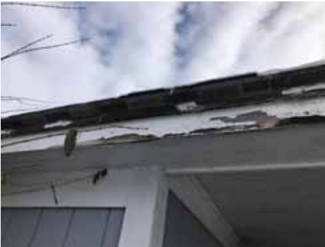
2.21: Deteriorated wood trim at modulars
