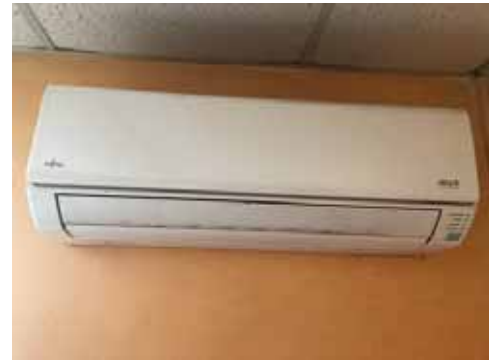
4.15: Modular classroom – ductless AC unit
