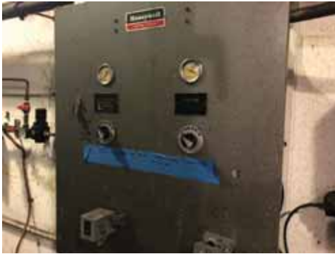
4.19: Pneumatic control panel
