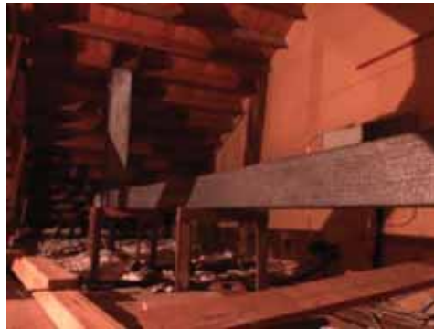
4.14: Attic – Exhaust ductwork
