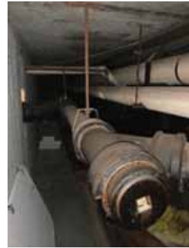
6.15: Cast iron piping in crawl space
