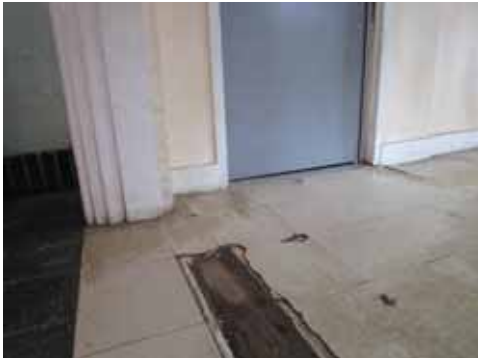
3.30: Uneven, damaged threshold between corridor and modular wing
