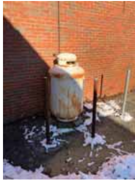
6.14: Exterior Propane Tank
