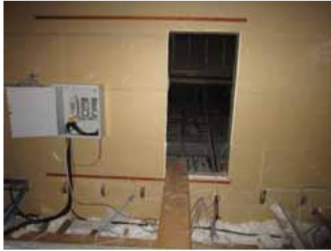
3.36: An opening has been cut in the attic firewall
