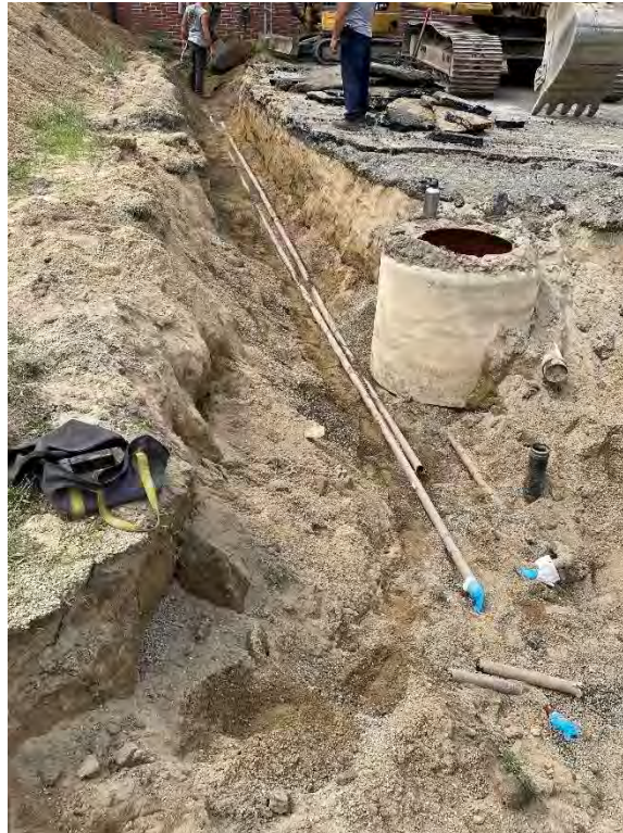
Photo 3: View of feed/return lines from tank to building.
